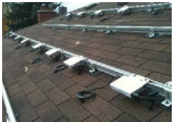
A Solar Electric Racking System
