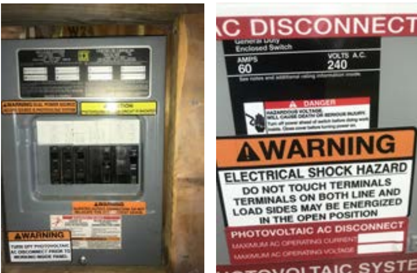
Photo 11: AC disconnect/load center manufacturer's label obscured: NEC 110.21
